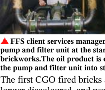
▲ FFS client services manager Carl Frankenveld at the offloading pump and filter unit at the start of the fuel system for the brickworks. The oil product is offloaded from road tankers through the pump and filter unit into storage tanks
