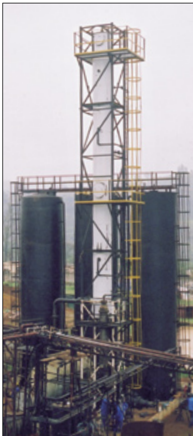
▲ New distillation column and ancillary plant being constructed in Pietermaritzburg for toll solvents and specialised chemicals processing.
