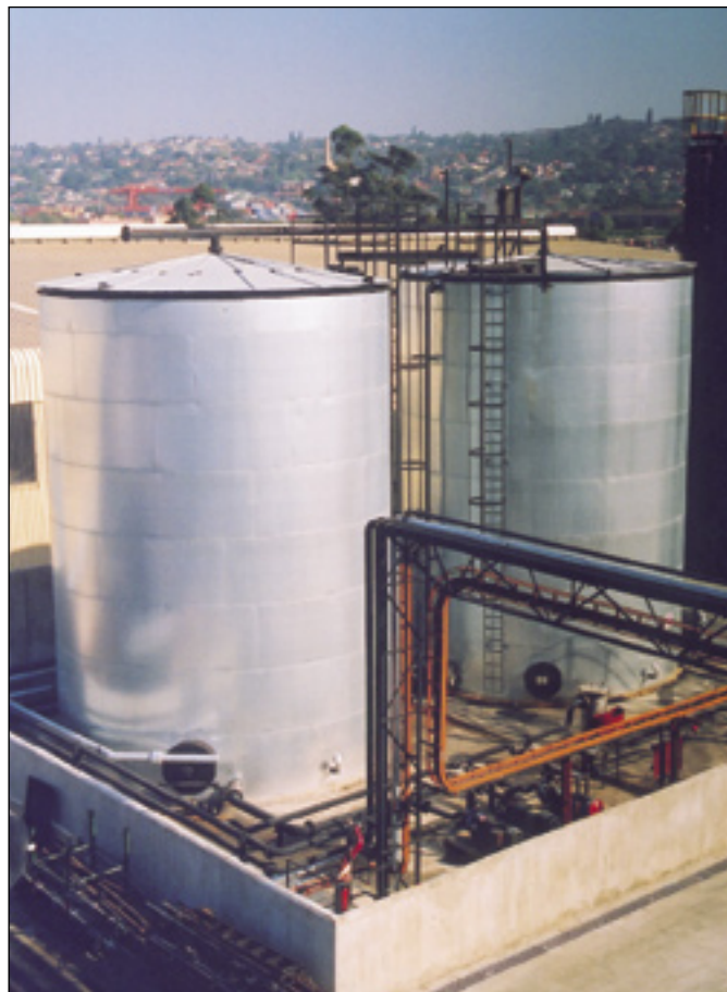
▲ Final product tanks at the Durban factory.
