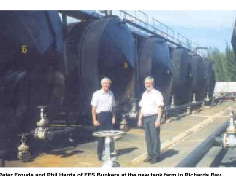
Peter Froude and Phil Harris of FFS Bunkers at the new tank farm in Richards Bay.
