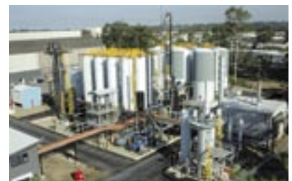
▲ Overview of plant and storage tanks at the Australian refinery
